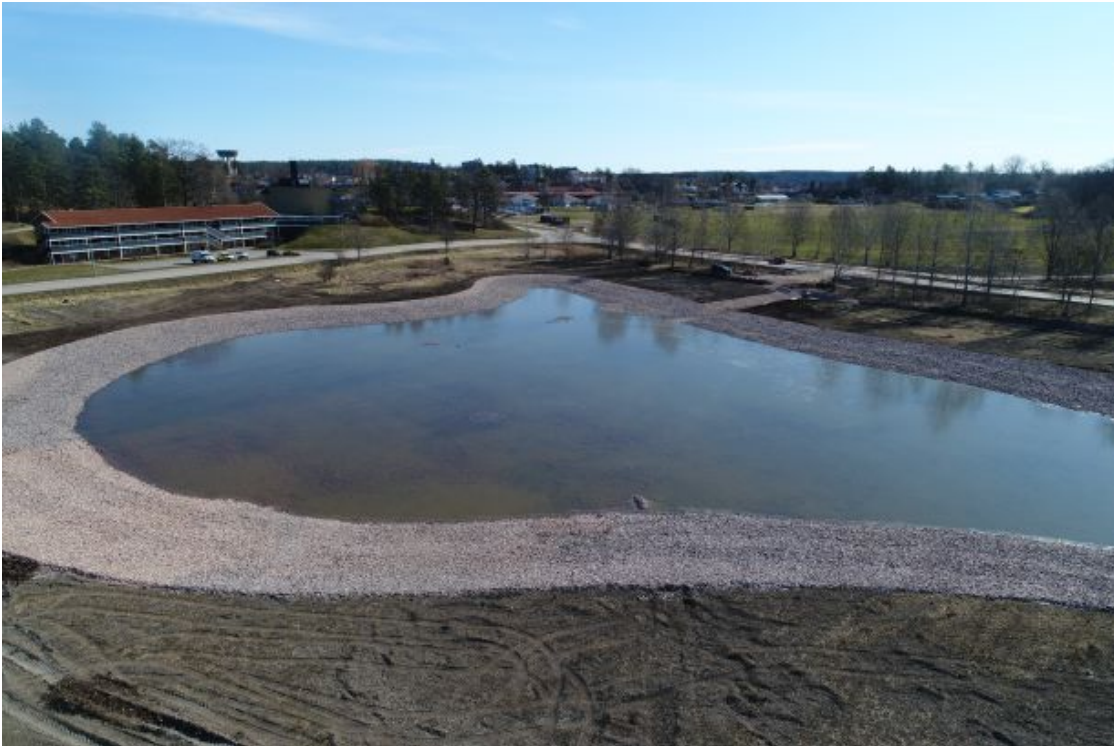
Newly constructed Stormwater dam with multiple functions close to Gamleby constructed 2019-20. The multiple functions are Nutrient retention, Irrigation, Discourage flooding, Recreation area.
